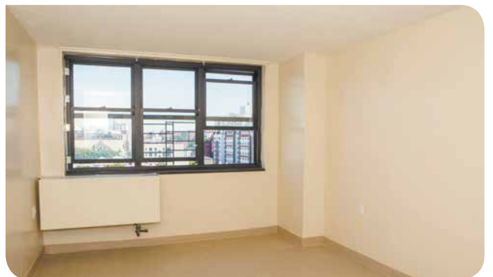
All apartments now have new windows and screens, plus air conditioning and heating units that tenants can control themselves.
